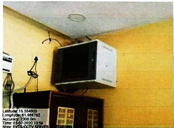
CCTV SERVER ROOM
