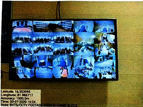
CCTV CONTROL UNIT
